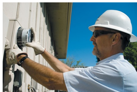
Smart meter installation
