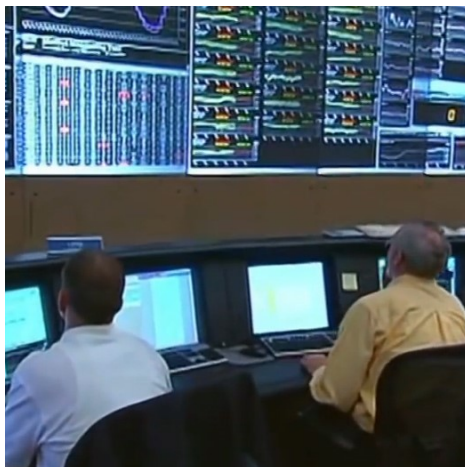
MISO control room
