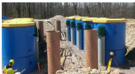
Beacon Power storage facility, Hazleton, Pa. Source: Department of Energy
